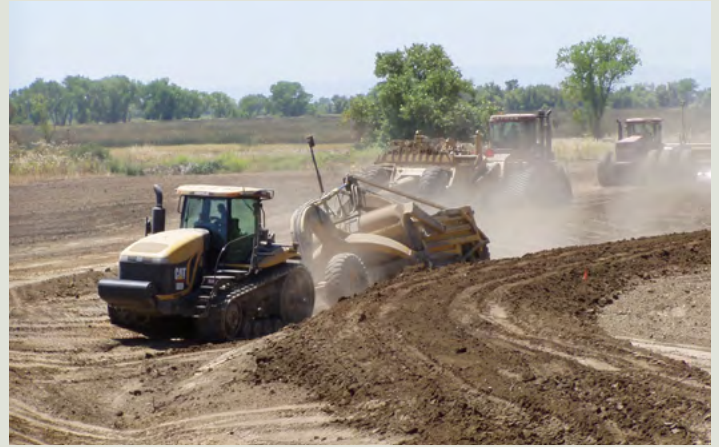
Levee construction for wetland habitat restoration, Gray Lodge Wildlife Area - Ducks Unlimited, Inc.
